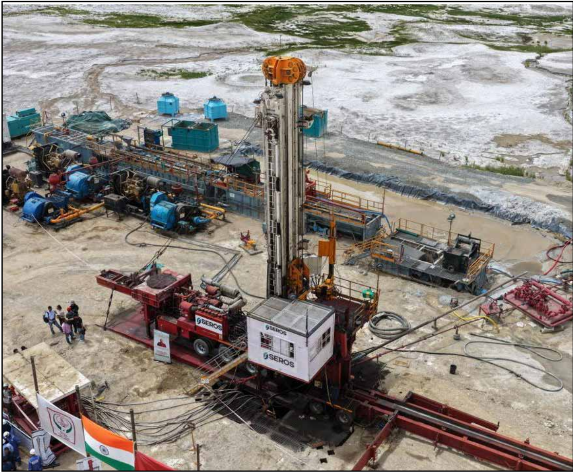
Photo Caption: Geothermal wells at Puga valley in Ladakh.
