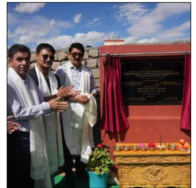
Chairman/CEC, LAHDC, Leh, Adv. Tashi Gyalson, ceremoniously laid the foundation stone for the construction of a new Culture Centre and Dharmasala for Tashi Lhunpo Monastery, Leh marking a significant milestone for this important project.
