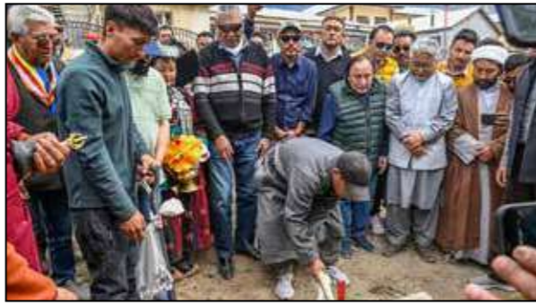
During the ground worship ritual (Bhumi Pujan) at the new construction site of the Buddhist Gonpa in Kargil.
